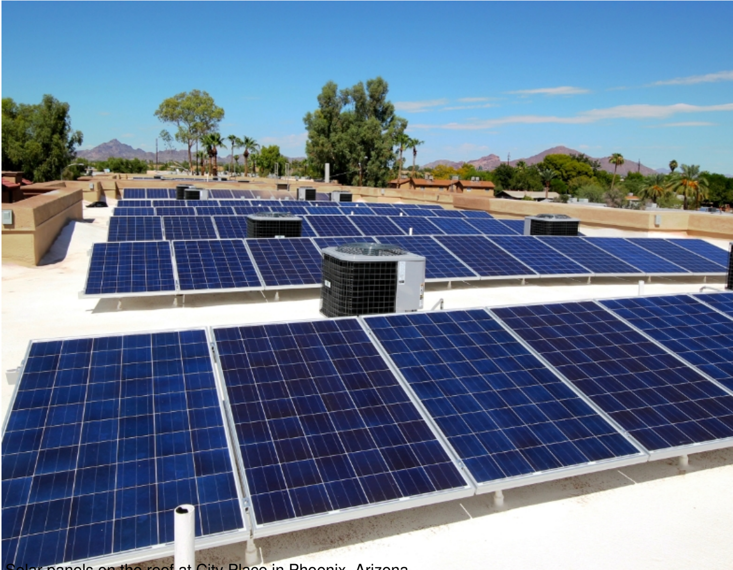
Solar panels on the roof at City Place in Phoenix, Arizona.
